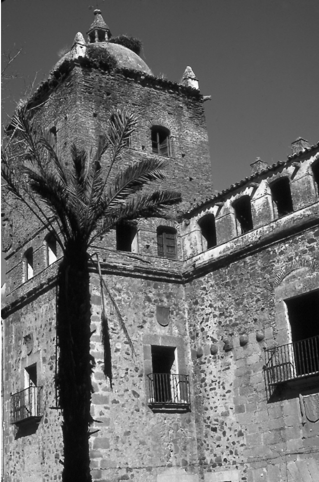
Figure 6.1. Palacio de los Toledo-Moctezuma, Cáceres, Spain, prior to restoration. (Photo courtesy of Ida Altman.)
